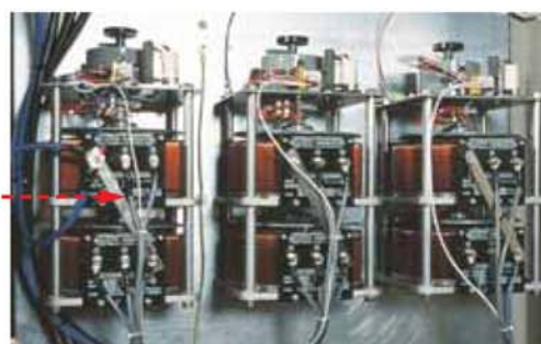
Motorised variable autotransformers Fig. 7
